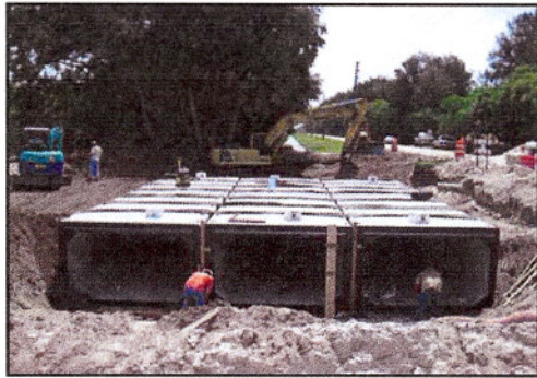
Figure 1. V.A. Paving Installed a Triple Barrel Run of 6-ft X 10-ft Precast Reinforced Concrete Box Culverts.
