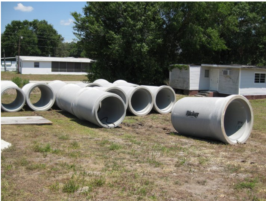
Figure 5. 48-inch diameter reinforced concrete pipe will replace a failing corrugated metal culvert.
