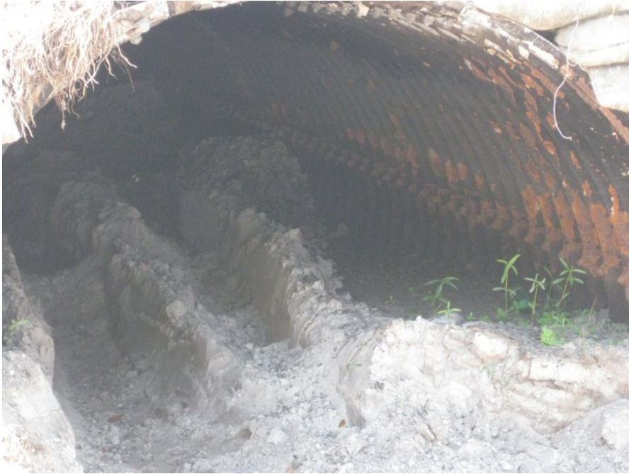
Figure 2. Corrugated metal pipe deteriorating along Canoe Creek Road in Osceola County, Florida. This CMP appears to have been originally bituminous coated.
