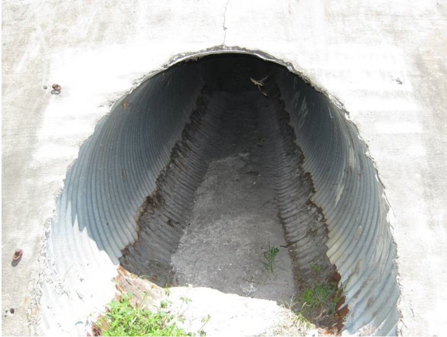
Figure 4. Invert deterioration in corrugated metal culvert.
