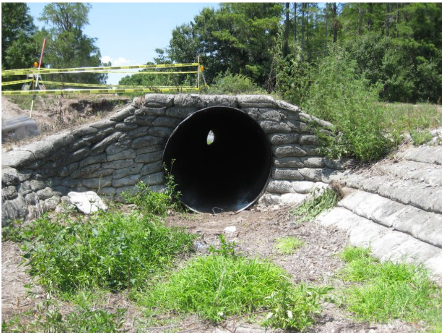
Figure 3. Corrugated metal pipe to be replaced. The pipe has become egg-shaped.
