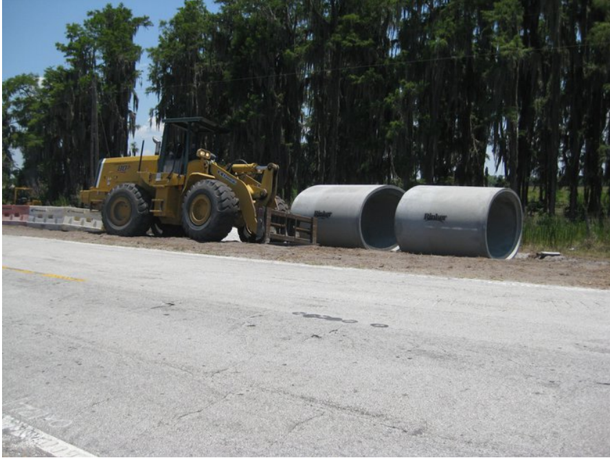
Figure 6. 63x98 HERCP to replace failing corrugated metal culverts along Canoe Creek Road.
