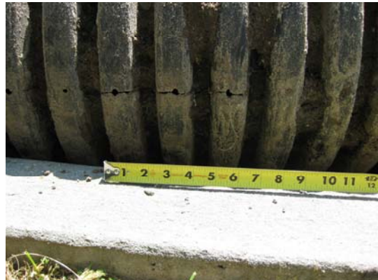
Figure 4. Longitudinal cracks developed through HDPE corrugation pierce punch holes.
