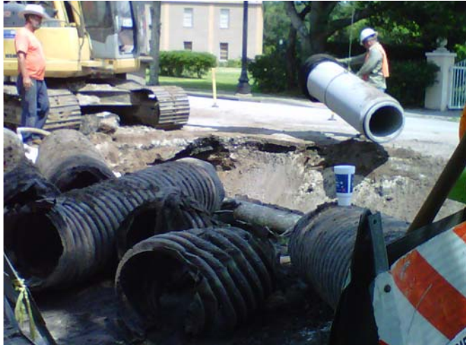
Figure 1. 18-inch ASTM C76 Class III RCP replaces less-than 15-year old corrugated HDPE pipe.
