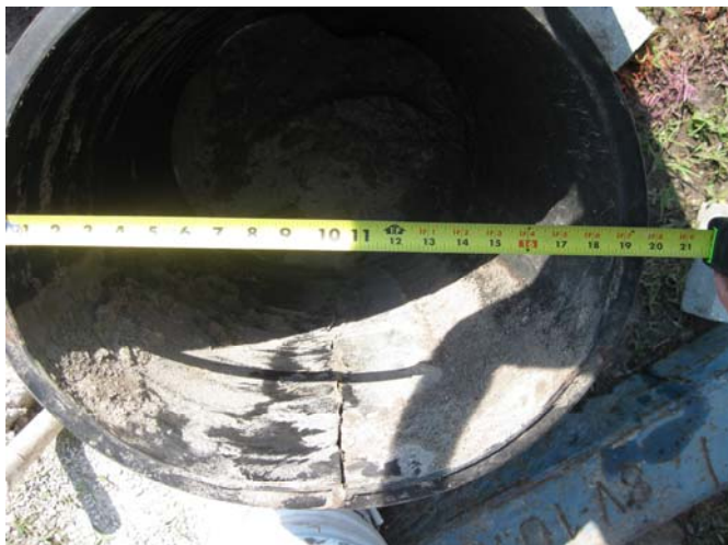
Figure 2. Upon excavation, some of the 18-inch HDPE pipe remained deformed, with horizontal dimensions of 19 to 20 inches and cracks along the invert.
